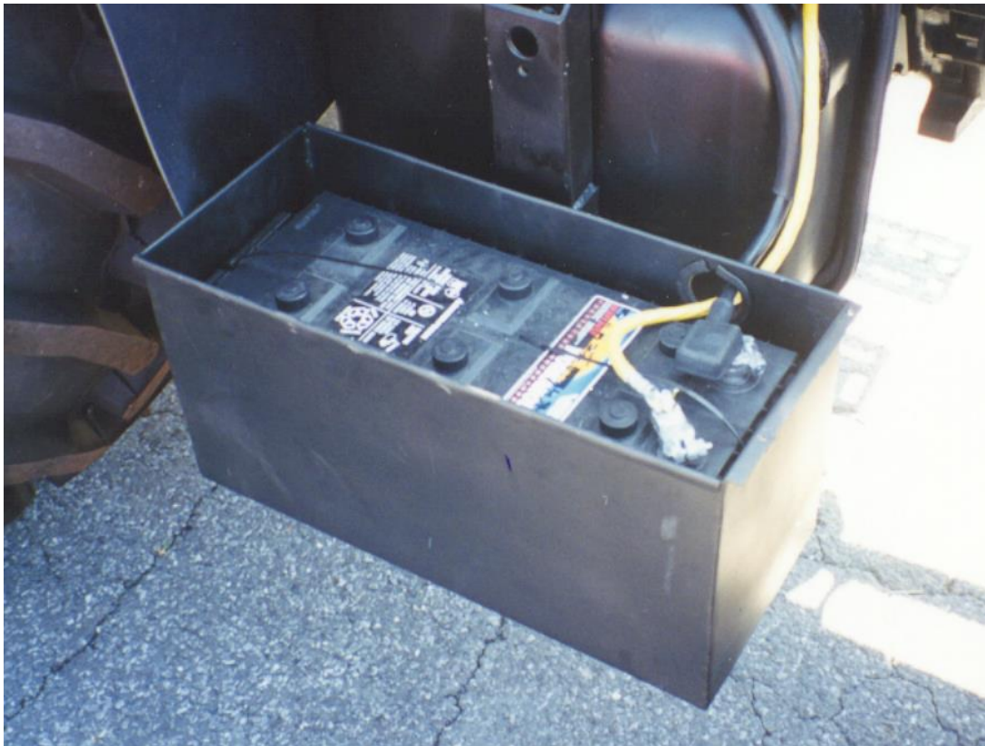
Battery in place in box.
